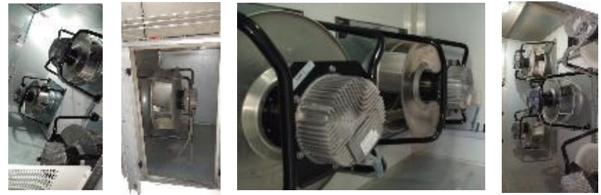
EC fans for AHUs, UFADs, Exhausts, DOAs
